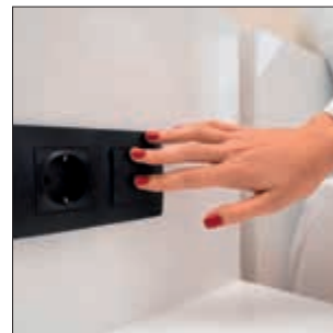
The colour temperature change in steps can also be set using the switch.
